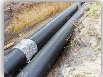
Pipeline Leak Detection System
